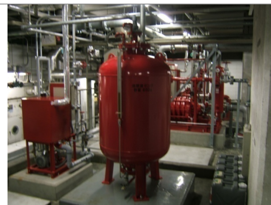
Fire fighting system for underground parking (400L tank)
